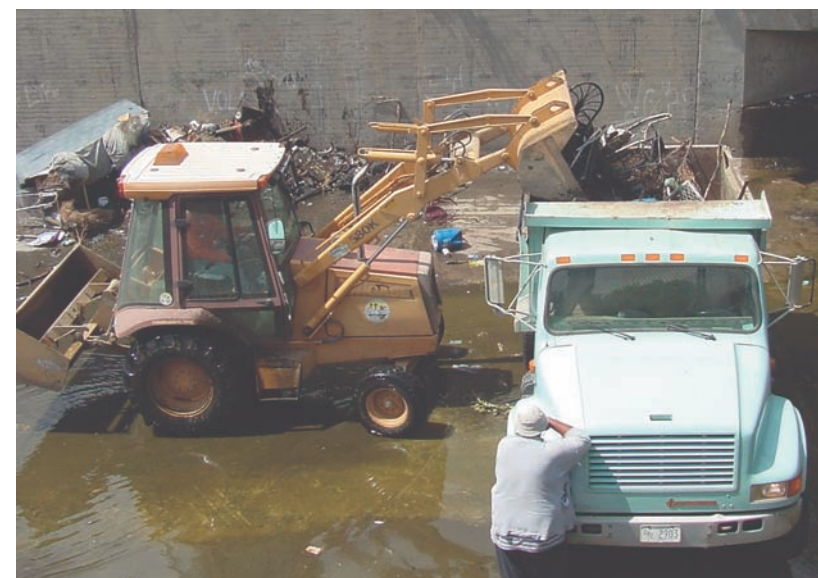
Heavy equipment was brought in to deal with larger pieces of debris.
